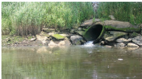
Storm drain outfall at Moody Lane. Photo: Earthplace.
